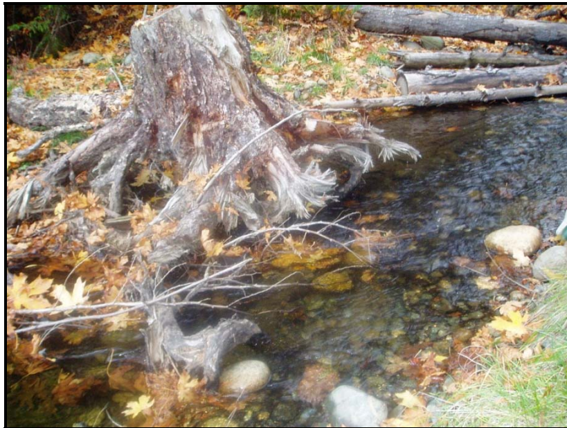
Photo 5. Example of large woody debris installed near Station 3 on the C.W. Young Channel to create habitat for juvenile salmonids.
