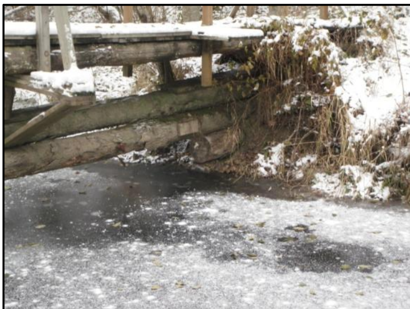
Photo 6. Site conditions at the foot bridge of the MB Channel near station 4 on 24 November 2010.
